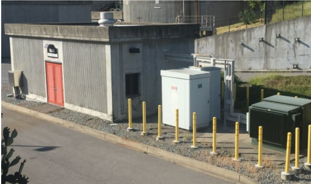
Switchgear building and transformer
