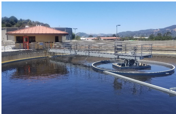
Secondary clarifier in operation
