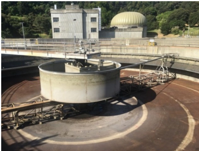
Secondary clarifier internal equipment
