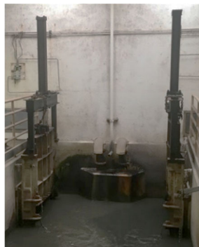
San Rafael and Ross Valley influent gates
