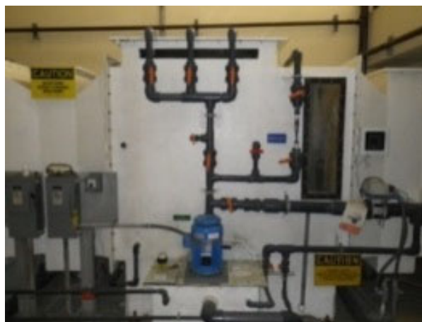
Solids Handling Building odor control scrubber
