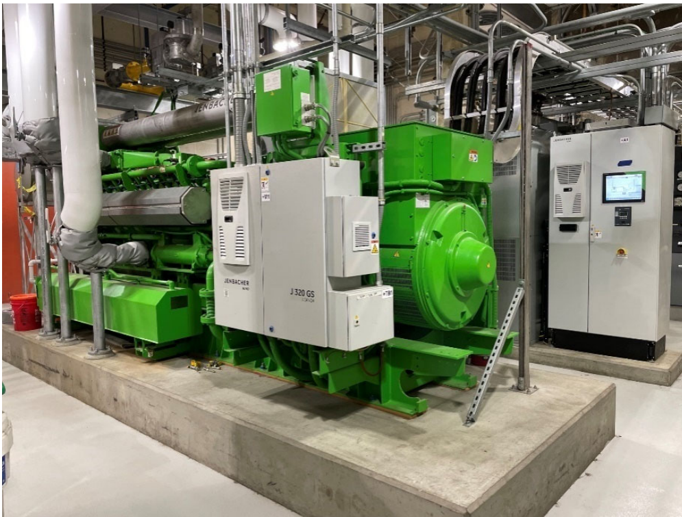
New cogeneration system
