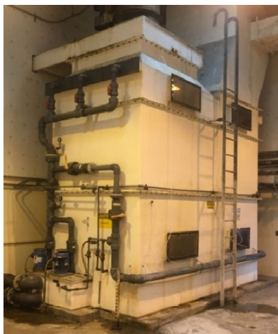
Headworks odor control scrubber
