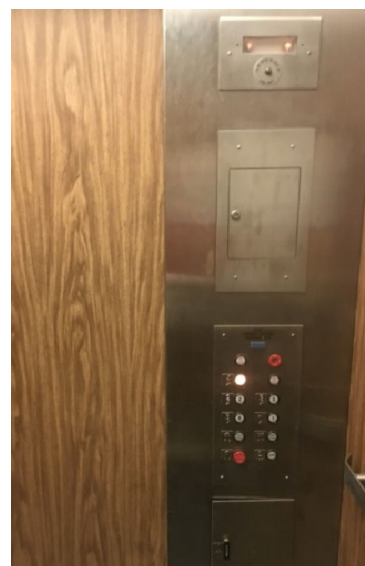
Elevator Control Panel
