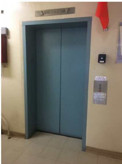
Solids Handling Building Elevator
